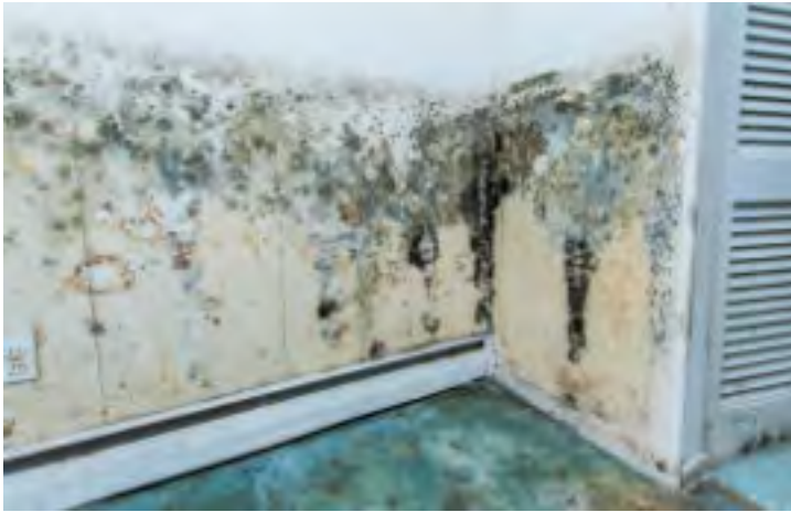
Figura 4.2 - Edificio danneggiato dall'acqua e contaminato da micromiceti (WDB); fonte: https://www.nbcnews.com/health/health-news/sick-building-fungi-release-toxin-directly-air-study-finds-n776126
